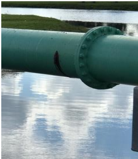
Figure A.5.2 - Damage to 24" DIP on December 29, 2016
