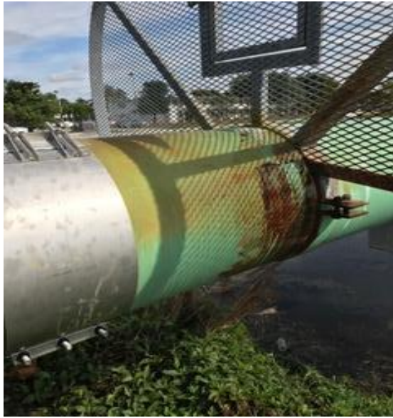
Figure A.5.1 - Damage to 24" DIP on December 21, 2016
