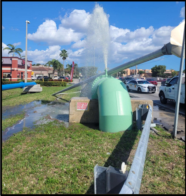
Figure 1 - Picture of Car Accident which caused Spill Event on February 19, 2022
