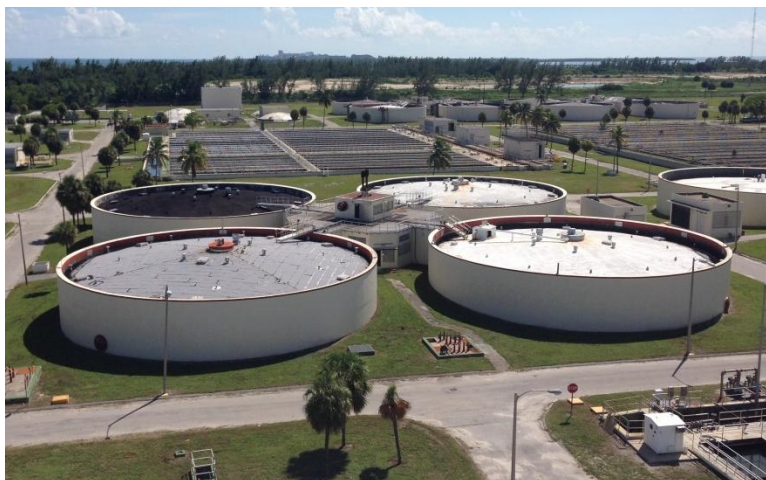
Figure 1: Typical Digester Cluster Configuration
